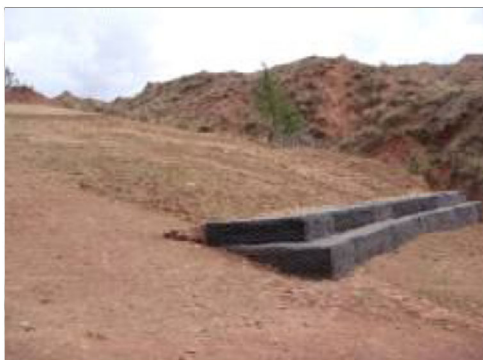
PLNG Transport System, Peru
